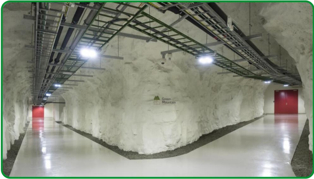
Located in a former NATO munitions bunker, the Green Mountain data centre leverages an adjacent fjord for cost-effective, sustainable cooling. Photo courtesy of Green Mountain – Photographer: Knut Bry
